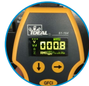
Displays neutral to ground voltage
