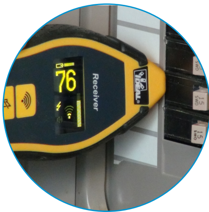
Finding Breakers or Fuses
