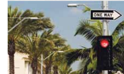
traffic signal controls
