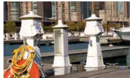
marine shore-power and dock lighting
