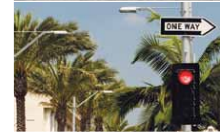
traffic signal controls
