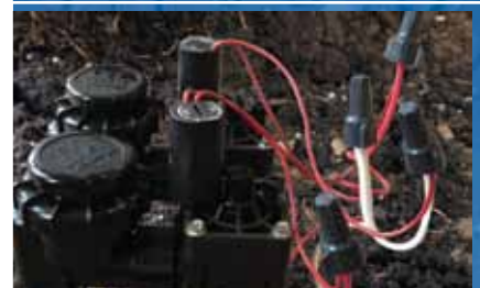
irrigation and sprinkler systems
